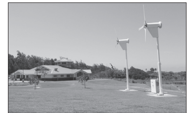
Two wind energy turbines help to generate electricity for North Kohala Public Library.
